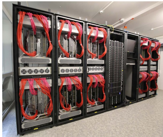
Figure 2. The BrainScaleS-1 machine room comprising 20 wafer modules organized in 5 racks. A slot in the middle of each rack hosts the analog readout module and the main control units of its neighboring wafer modules. Gigabit-Ethernet cables connect each wafer module via aggregation switches to the control cluster positioned in the middle rack. © [2017] IEEE. Reprinted, with permission, from [14].
